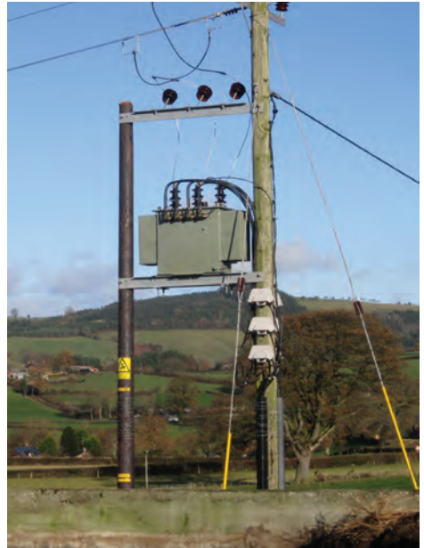
High voltage 3 phase supply and transformer
