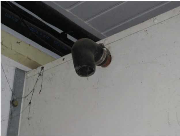
Overflowing hot water heater
