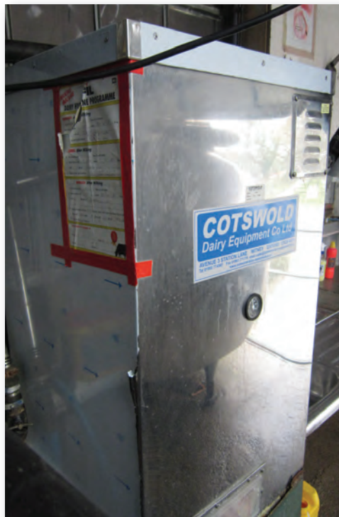
Hot water heater
