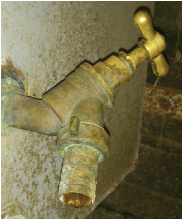
Leaking old tap
