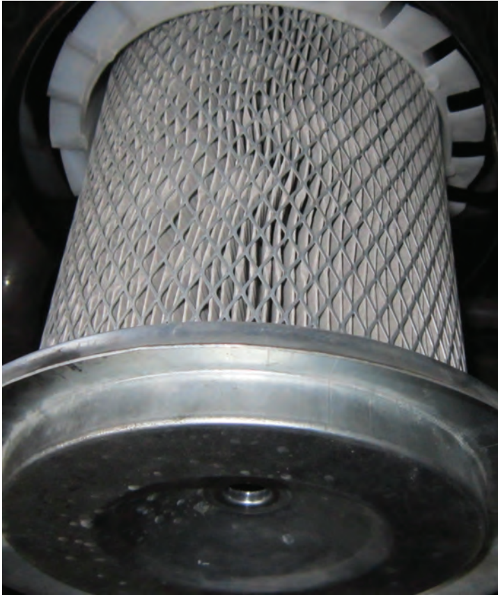
Ensure air filters are regularly cleaned
