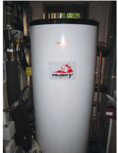
Hot water 'buffer' tank or thermal store
