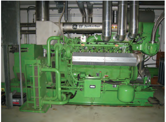
Combined Heat and Power (CHP) engine
